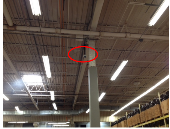
Picture B: One of several newly installed security cameras on FCPS' side of the Central Warehouse.
