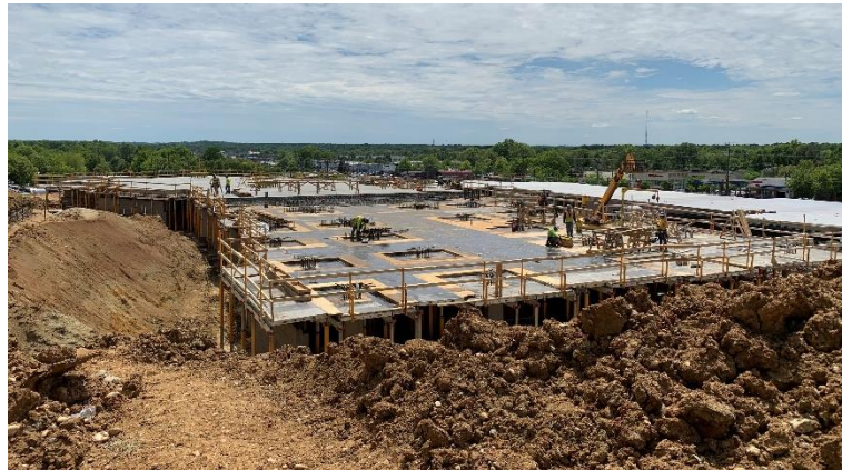
Pictured From Top to Bottom: Rendering of the Residences at North Hill Development; inside the garage of building 2A looking toward Richmond Highway; building 3A podium slab form work for slab placement.
