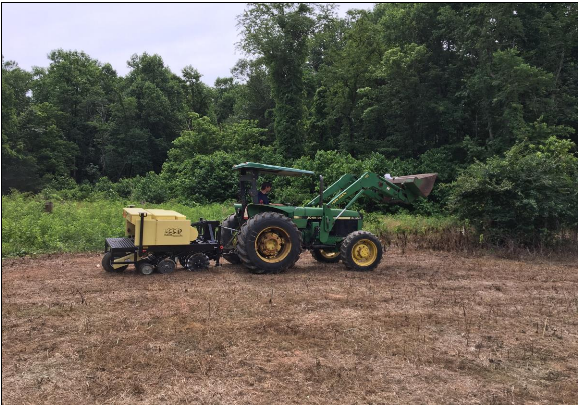
After bare-ground herbicide treatments, tractor raking, and leaf blowing, RB1 is prepared for restoration seeding (June 2019).
