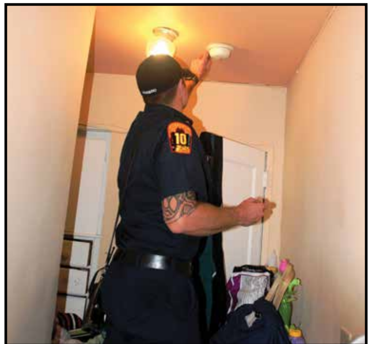
Preventing the 911 Call . . . firefighters install smoke alarms in homes throughout the county.
